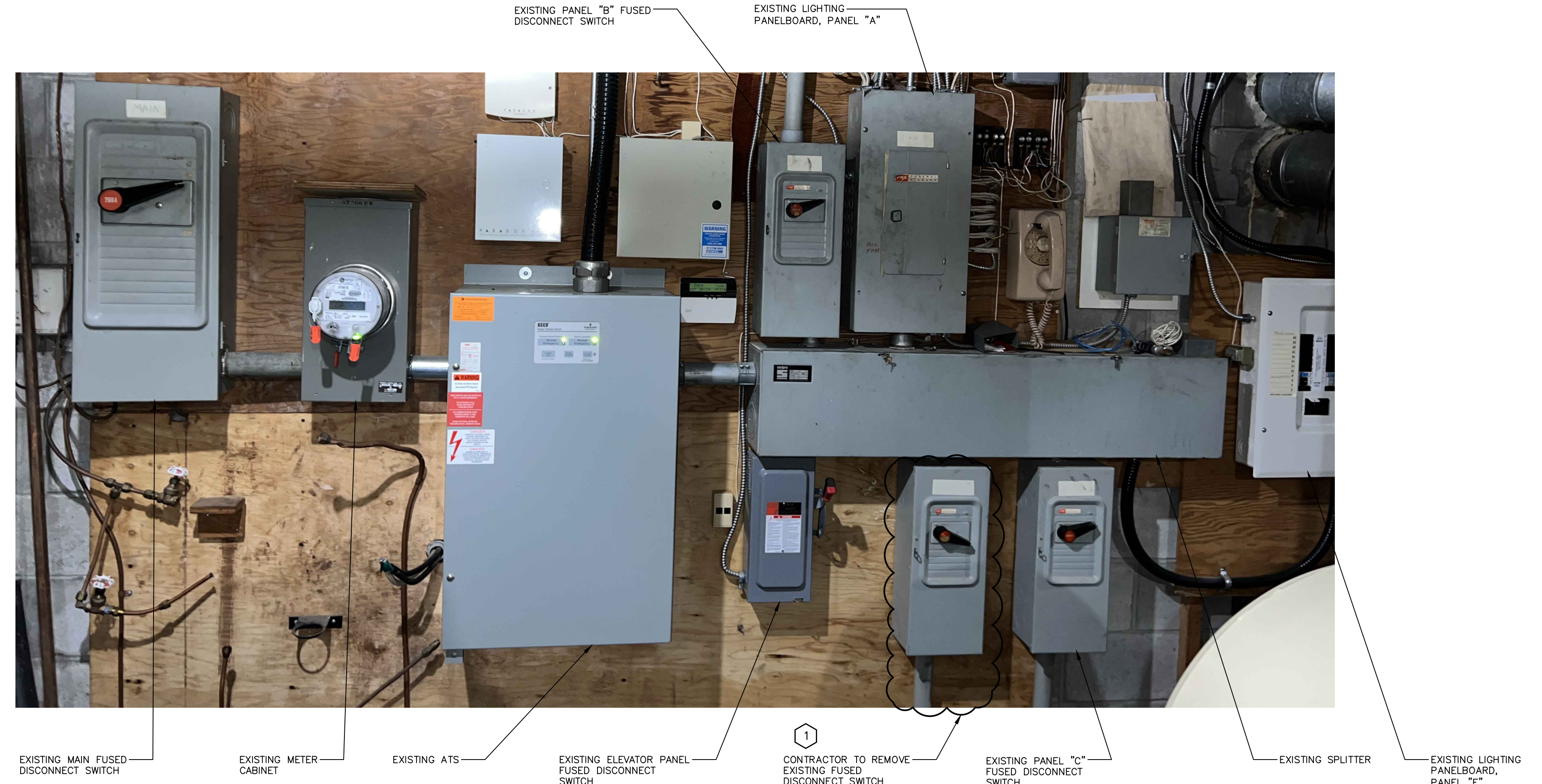
2 EXISTING POWER DISTRIBUTION IN SERVICE ROOM E2.1 - NTS
