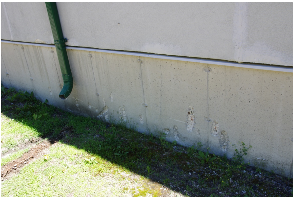
Photo 3 – South Side – Shrinkage Crack & Spalls / Damage
