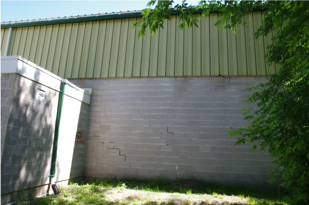
Photo 7 – Stepped Cracking just East of Zamboni Room – South Wall
