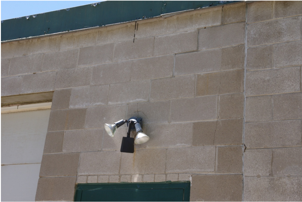
Photo 10 – North Side – Stepped Cracking
