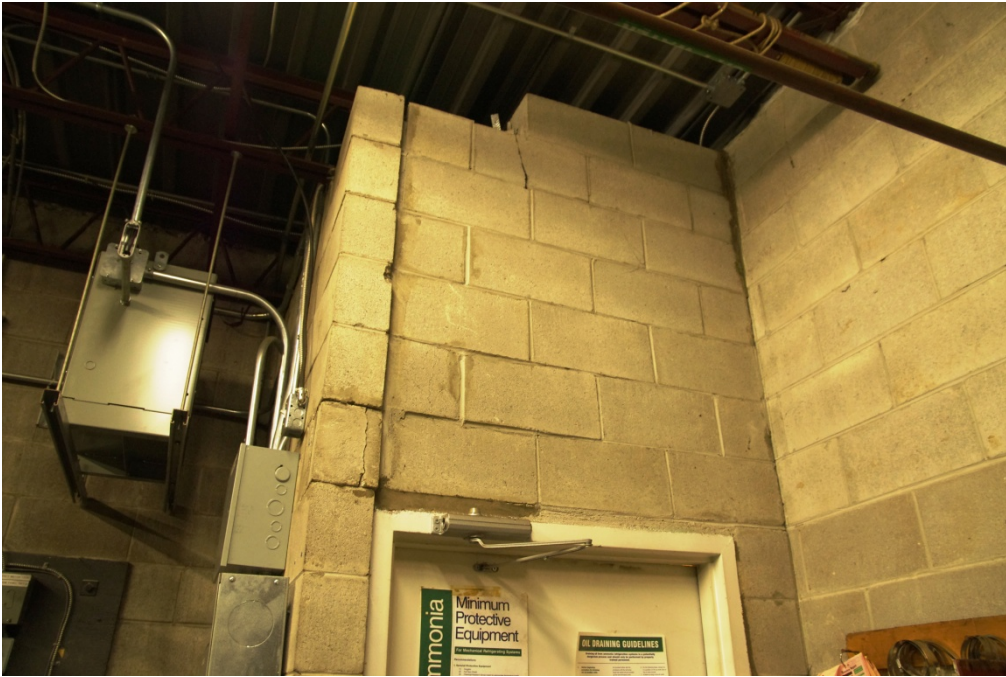
Photo 12 – Plant Room – Damaged Block Adjacent to Man Door
