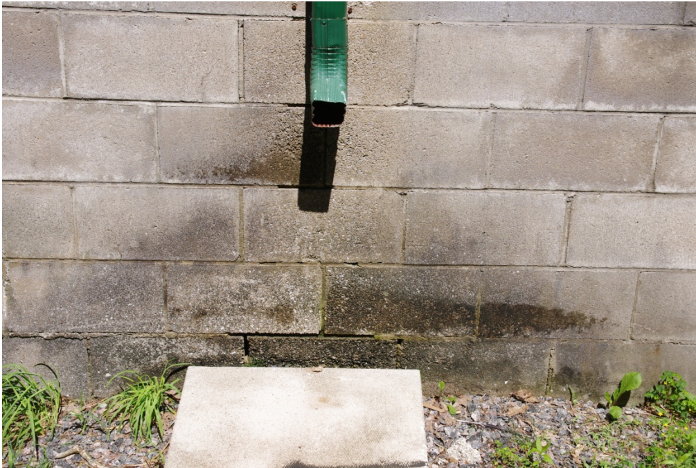
Photo 8 – East Wall – Eroded Block at Downspout
