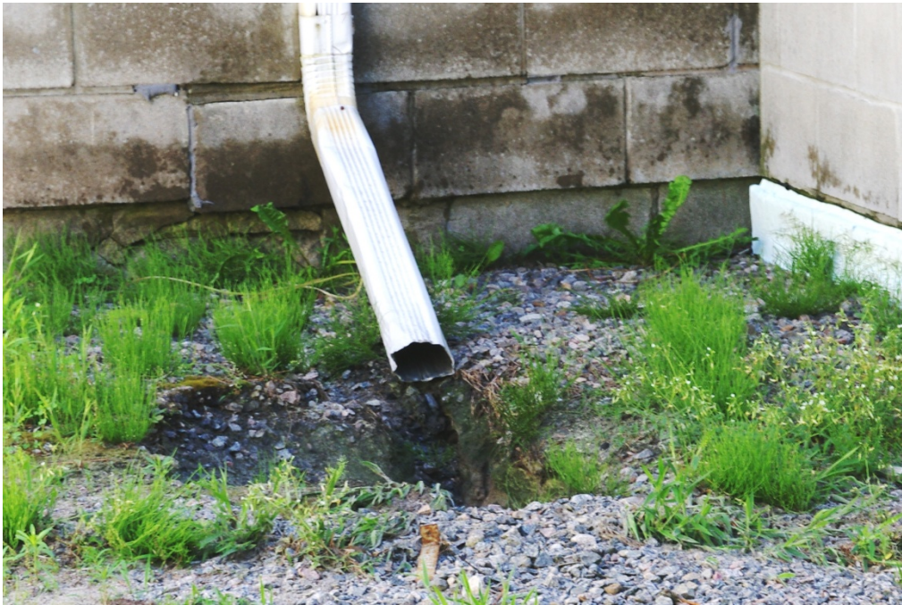
Photo 6 – Damaged Block & Erosion Adjacent to Zamboni Room
