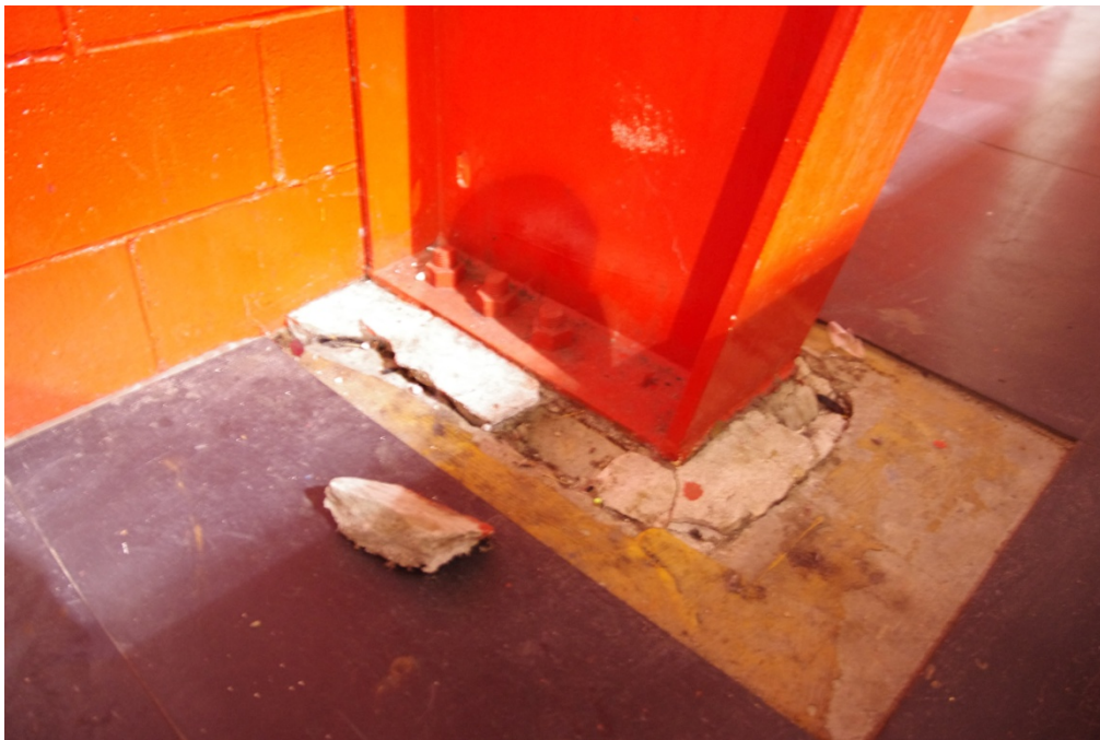
Photo 13 – Rigid Frame Base Plate with Cracked Grout on Pier
