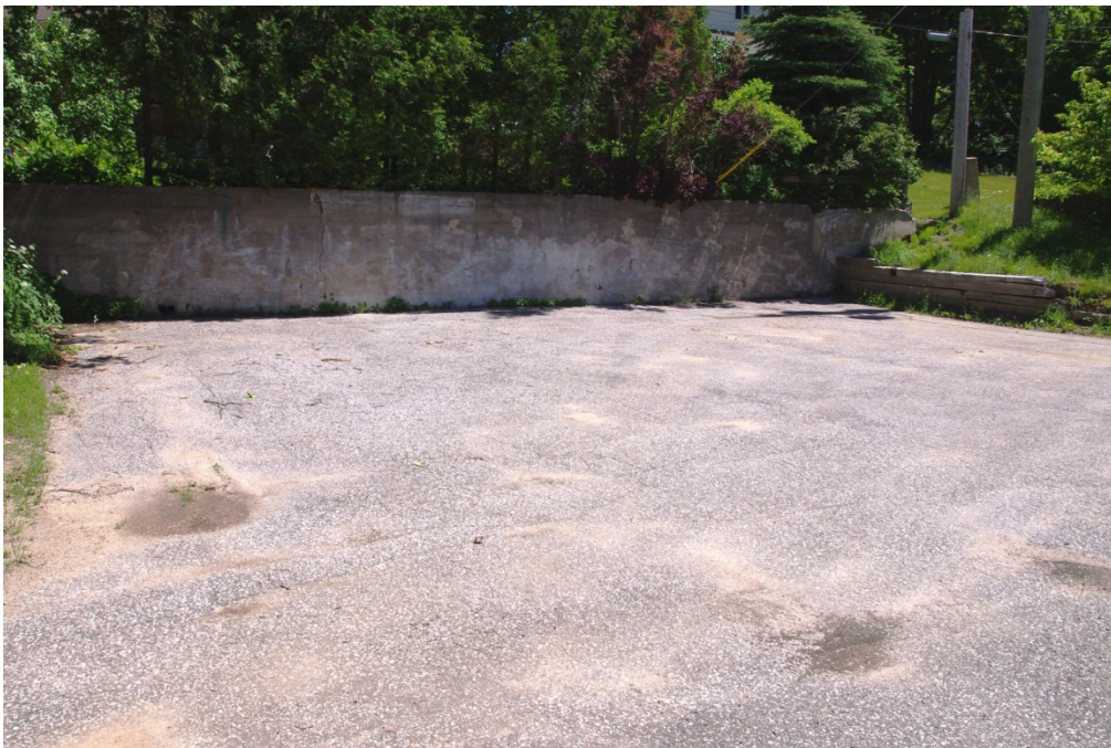
Photo 9 – North Side – Deteriorated Retaining Walls
