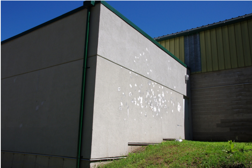
Photo 4 – North End of South Side Addition – Vandalism to Stucco Finish
